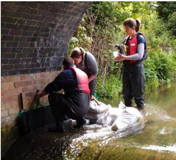
Installing an eel pass with our partners, North West Kent Countryside Partnership on the River Darent. © Joe Pecorelli/ZSL
